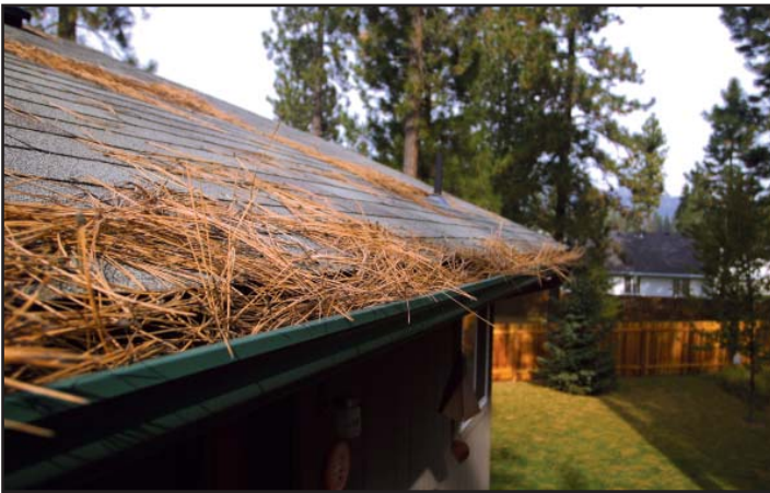
Remove debris from gutters and roofs.
